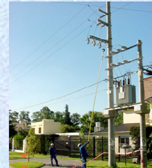
CT1: aerial MV/LV
