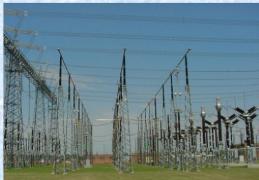
SE1: Substation HV/HV
